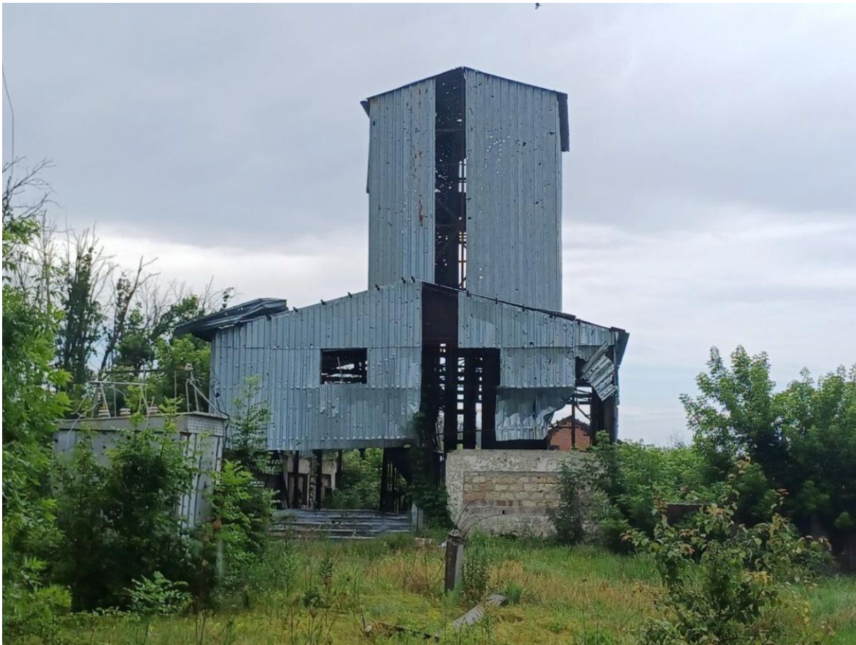
Picture 1. Illustrative picture of destroyed infrastructure in Kharkivska oblast
