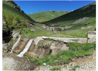
Water drainage system in Meghradzor
