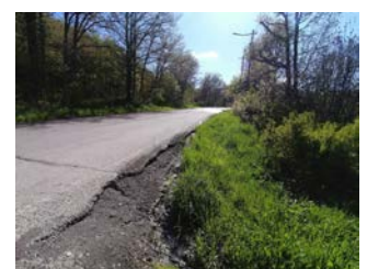
Landslide near Tsaghkadzor
