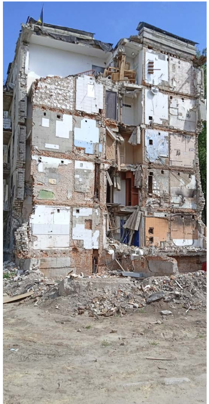
Image 2: Damaged housing in Kharkiv, July 2024 (REACH field team)
