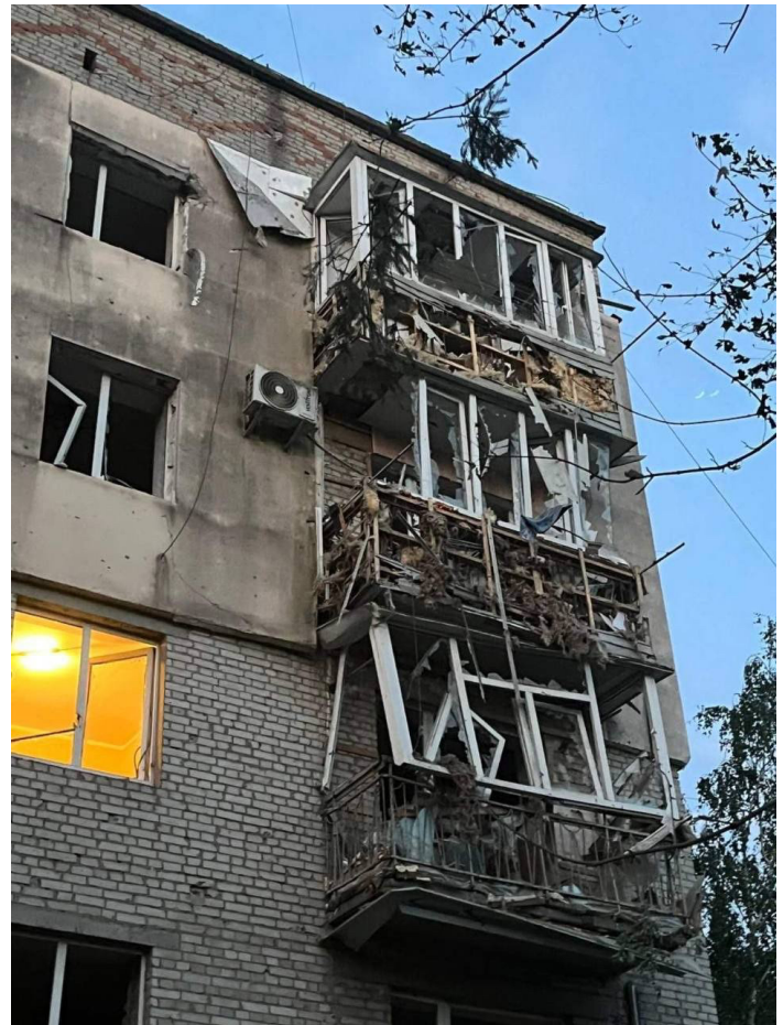
Photo 2: Damage to an apartment block in Sumska Oblast
