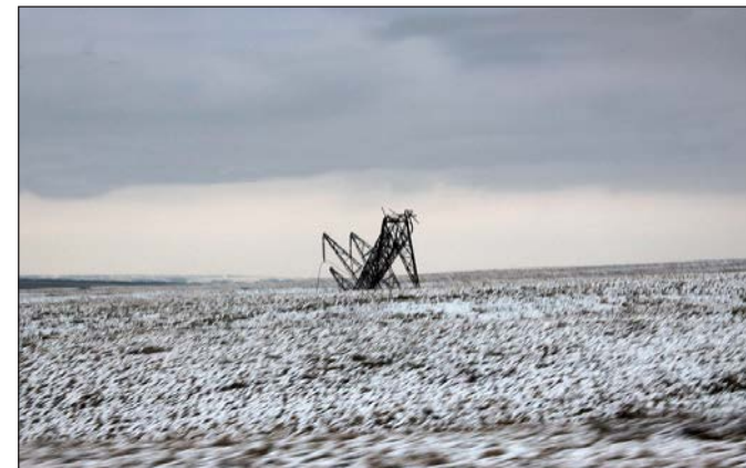
Damage of high-voltage power line near Granite, 27.11.2015. By Ministry of Defence of Ukraine.
