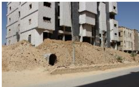
Figure 15. External perimeter of the building above the alternative underground hospital (after protective wall was built)
