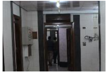
Figure 27. Electrical switchboard in the alternative underground hospital
