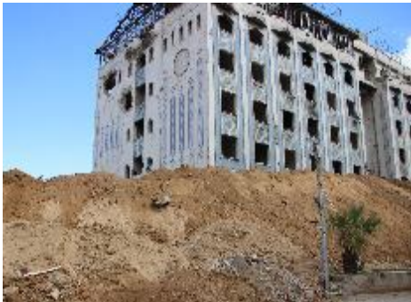
Figure 1. Protective wall around the perimeter of the building above the functioning underground hospital
