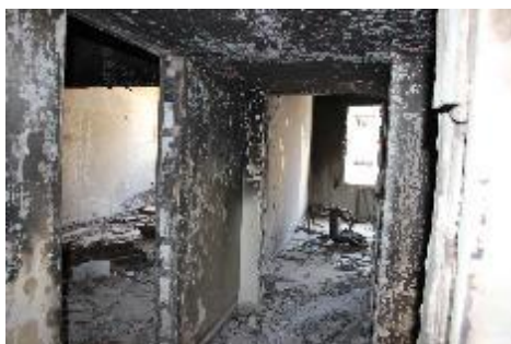
Figure 8. Second floor of the building above the functioning underground hospital (before reinforcement)
