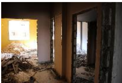
Figure 6. First floor of the building above the functioning underground hospital (before reinforcement)
