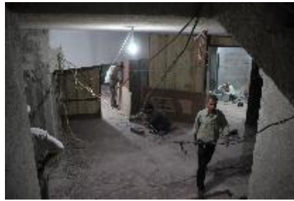
Figure 26. Overview of the electrical wiring within the basement area
