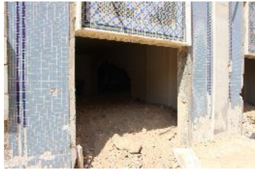
Figure 2. Extension of the earth used for the protective wall into the ground floor of the building above the functioning underground hospital
