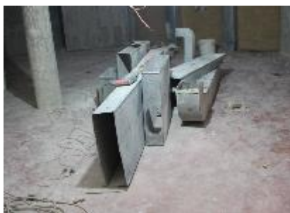
Figure 32. Pipes to be used for the ventilation system
