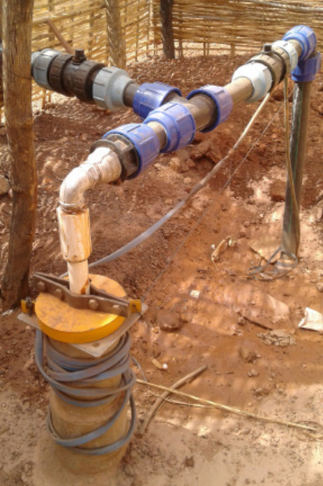
Figure 4: Generator operated borehole pump
