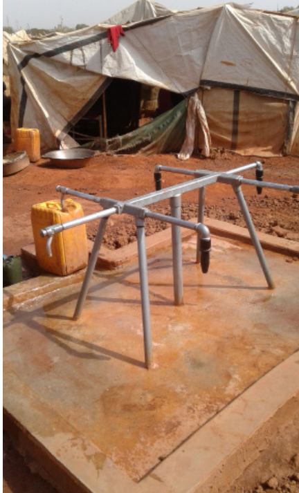
Figure 3: Water distribution point with six taps in Wau PoC
