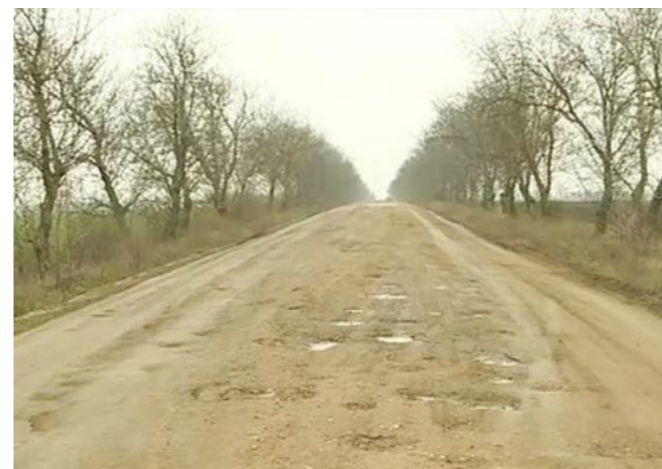
Road damage in Puhăceni, 12.01.2021
