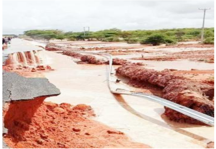
Damage to the Garissa-Modogashe during the 2023 flood. This disrupted access to goods, affecting livelihoods.
