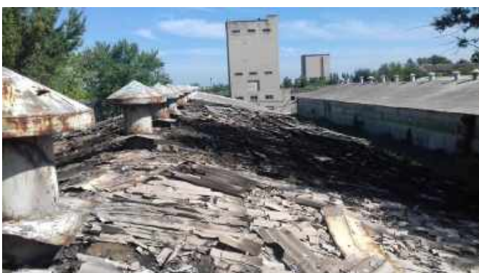
Fire damage at Bakhmut Agrarian Union, 03.08.2018 By State Emergency Service of Ukraine (SESU)
